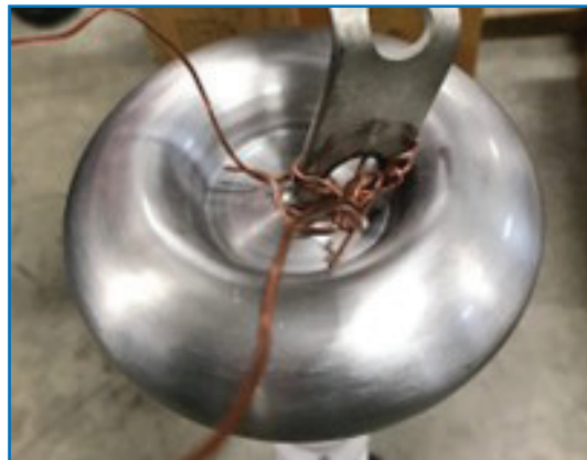
Figure 2. What Not To Do — Loose Wire Ends, Different Wire Thicknesses, Sharp Wire Bend.
